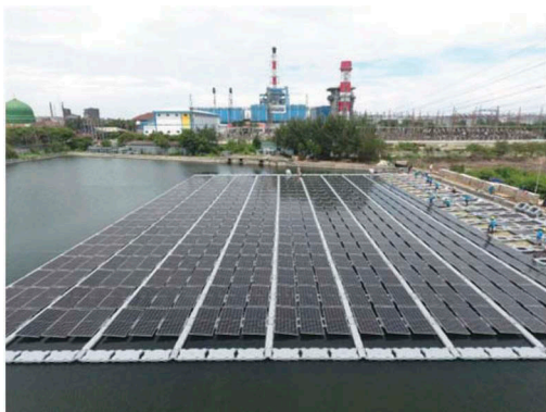
Figure 9. Floating solar PV plant installed on a pond in the Tambak Lorok, coastal area of Semarang (island of Java) (Meza 2023).
